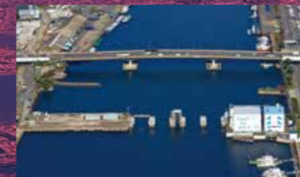
堀川口防潮水門 Tide gates at Horikawa River estuary
